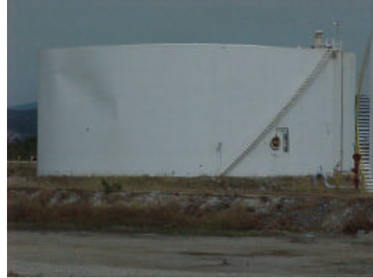
Figure 3. Steel cylindrical tank, which failed during hurricane Georges, 1998.
