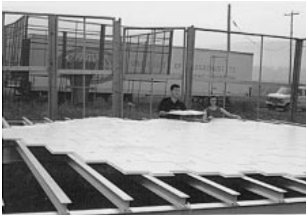
FIG. 4. TEP receive array under construction in the field. Clutter fences, the transmit horn, and the trailer are visible in the background.
