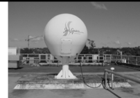
Antenna with radome
