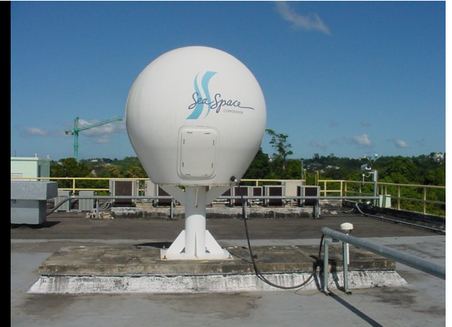
Antenna with radome
