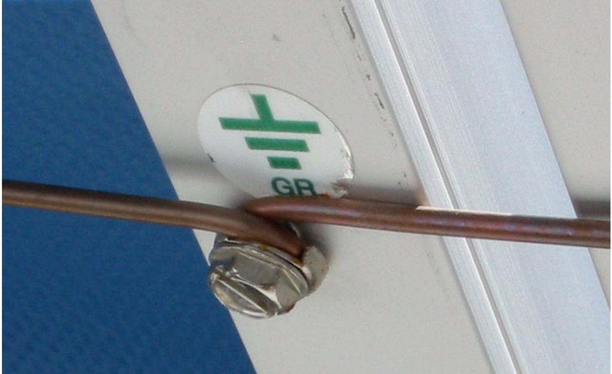
Figure G-2. Improper Module Grounding
